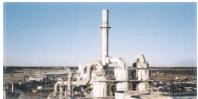
Sulfuric acid plant.
