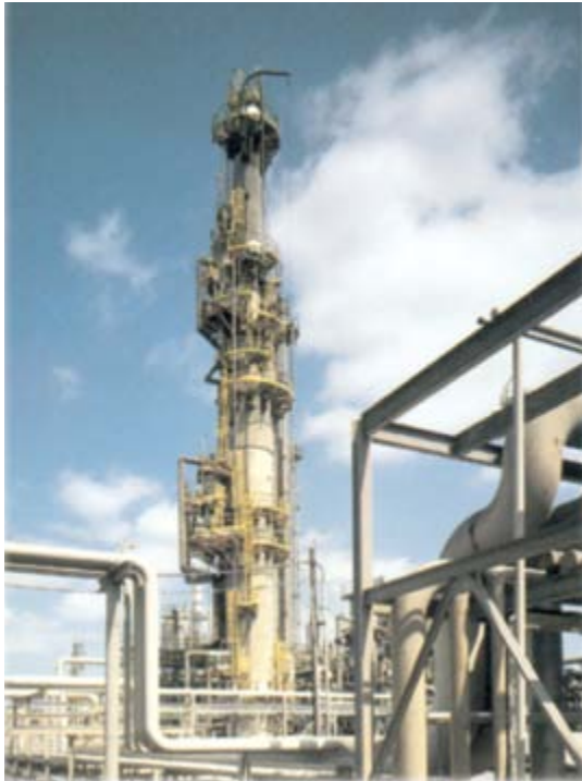
Fractionation tower in major USA refinery.
